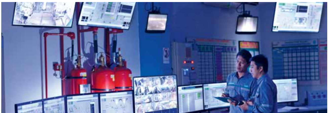
Ruang Kendali PLTU ANTAM ANTAM's CFPP Control Room
