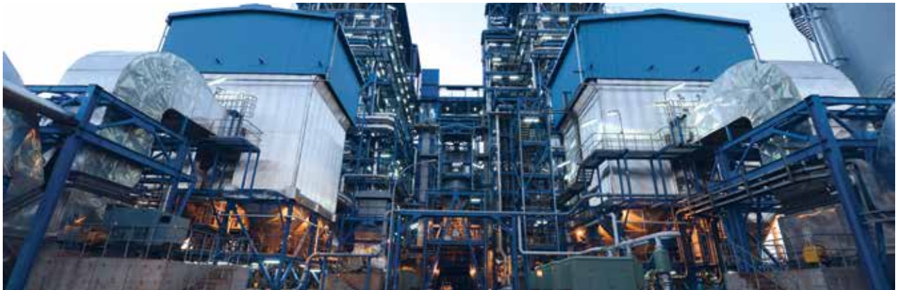
PLTU ANTAM di Pomalaa Berkapasitas 2x30MW The 2x30MW ANTAM's CFPP Facility in Pomalaa
